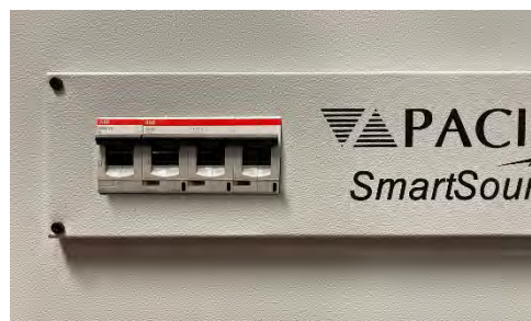
Figure 5-4: Mains CB in ON (upper) Position
